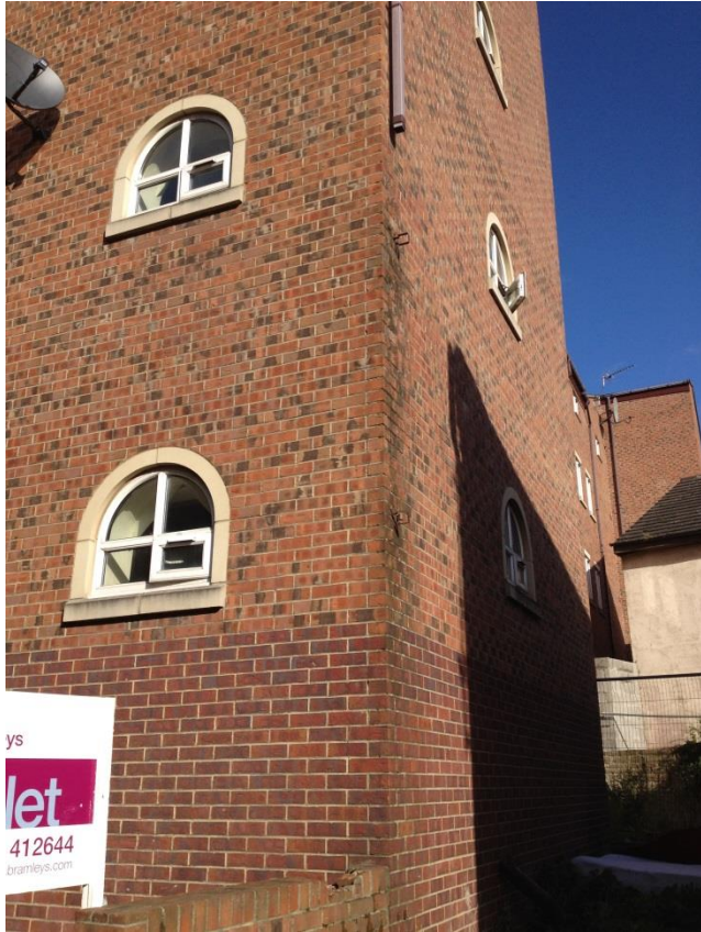
Missing drain down pipe 2 - Algae on walls
