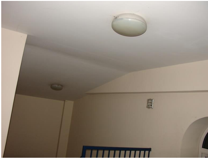
Broken light fitting 4 –Insides broken
