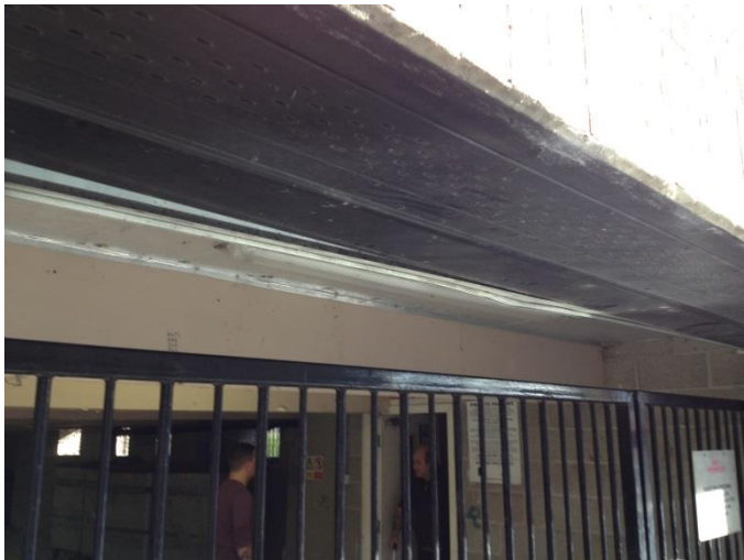
Gap above Gate – regularly used for access by youths and tramps
