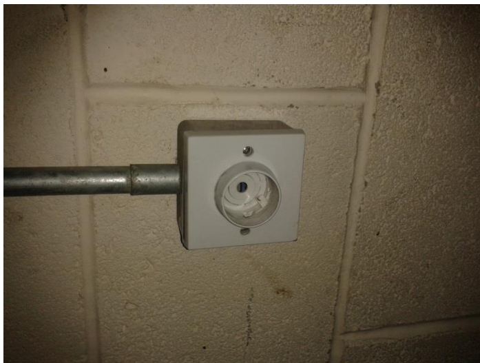
Broken light timer switch one of several
