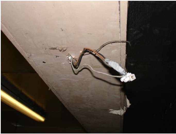
Exposed live wires 2
