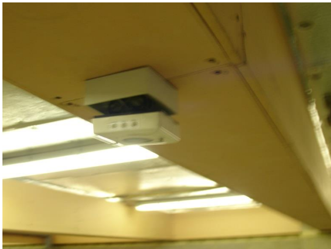
Broken Fire / Smoke Detector
