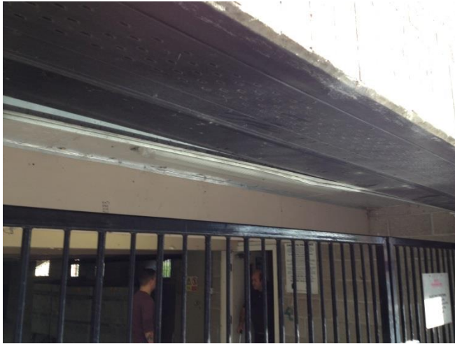
Gap above gate 2
