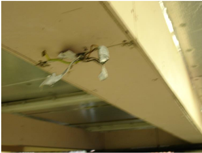
Broken light fitting 1
