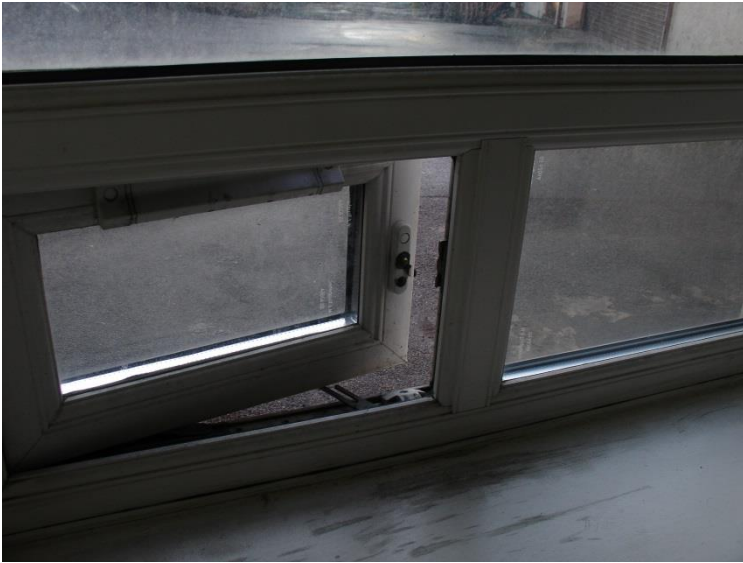
Broken window locks and frames
