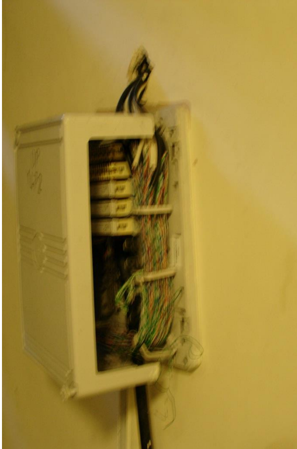
Damaged BT Box
