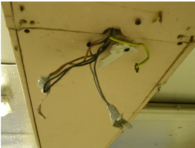
Exposed live wires 1
