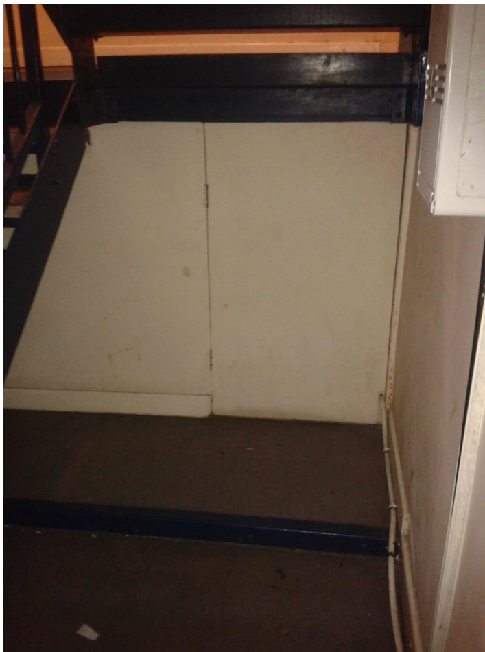
General cleanliness 1 and cupboard under stairs where tramps slept
